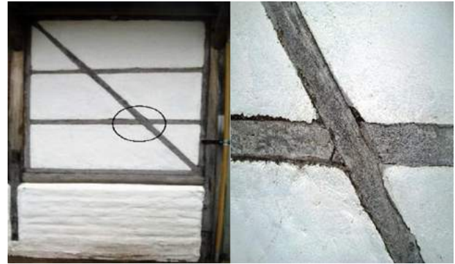
Fig. 14. Pathologies in joints on wattle and daub walls: a- Northern wall. b- Detail exterior joint.
