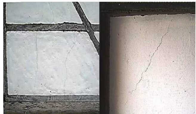
Fig. 15. Micro cracks on wattle and daub walls.
