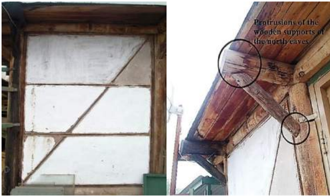
Fig. 12. Pathologies in front north-facing wattle and daub panels of the E.W.
