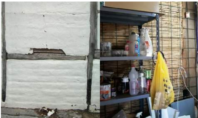
Fig. 13. Pathologies in south-facing wattle and daub panels, a-outside and b-inside surfaces.
