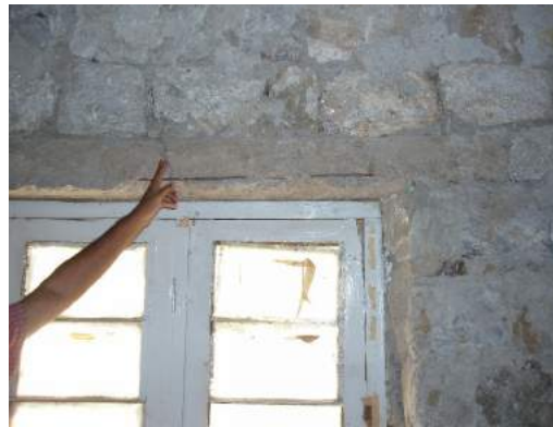
Broken lintel above the window
