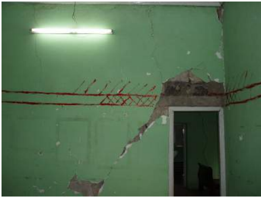
Major crack in center wall
