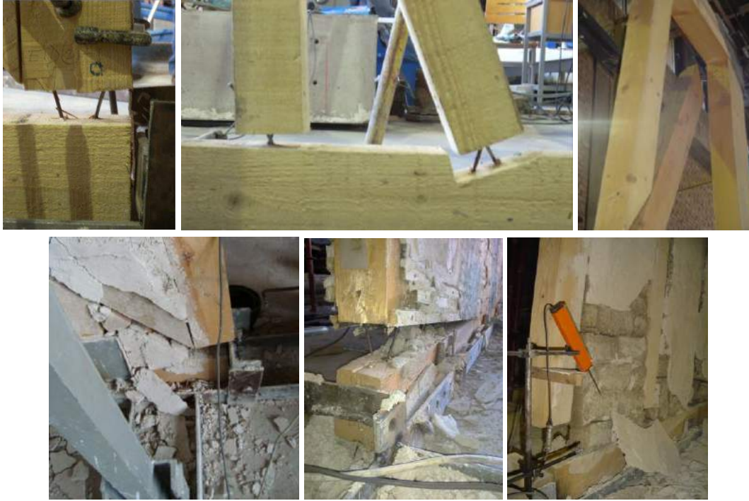
Figure 3. Failure at the nailed connections
