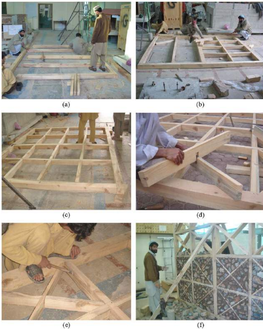
Figure 4. Various stages of dhajji walls construction: (a) Main frame of dhajji walls, (b) connecting horizontal elements, (c) complete dhajji frame without bracers, (d) connection of bracers, (e) nailing of the bracers, and (f) stone filling of the timber panels.
