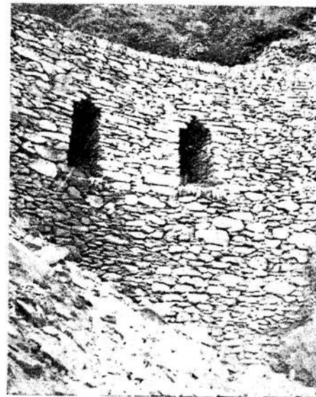
PHOTO 6. 7 m high dry stone masonry retaining wall with two Scupper openings at 3 m apart for cross drainage. Similar openings have also been provided for relieving seepage water pressures.
