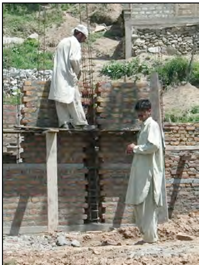
Fig. 5: To ensure proper filling of the tie-column it would have been better to fill the lower part of the tie-column together with the sill band
