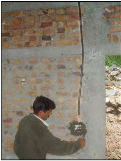
Fig. 15: No slits to be made in the masonry. Pipes can be hidden in the plaster, or left apparent
