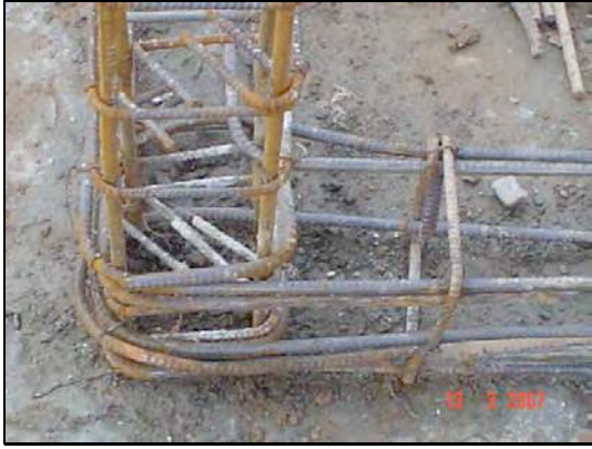
Fig. 13: Crowded corner reinforcement shouldn't have happened according to the drawings
