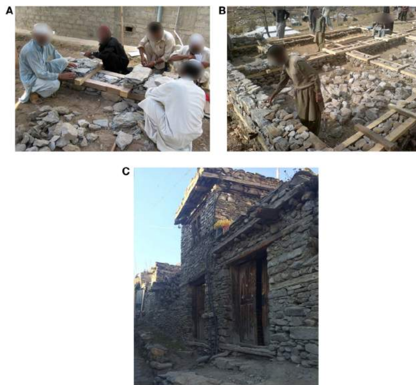
FIGURE 3 | (A) Construction process of a single Bhatar wall (by courtesy of the French Red Cross). (B) Construction of a Bhatar building (by courtesy of the Swiss Agency for Development and Cooperation). (C) A typical Bhatar building (photo credit: Tom Whity).
