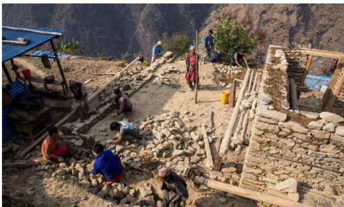
A practical session: the trainees are rebuilding a house during the training.
