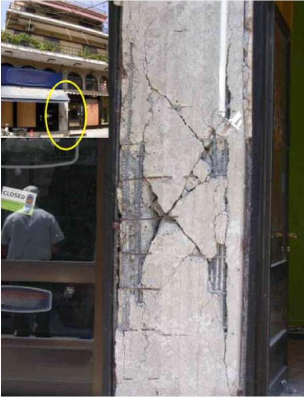
Fig. 11. Shear failure of ground floor column of R/C building (town of Lefkada). The non-existence of infill walls at the façade of the ground floor storey led to torsional phenomena.
