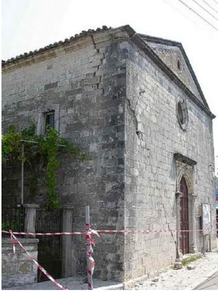
Fig. 14. Cracking of masonry walls of Agios Minas church (town of Lefkada).
