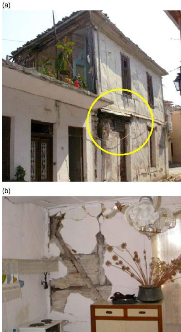
Fig. 9. Traditional dual system building in Lefkada town. (a) Local failure of stone masonry wall over door opening. Vertical loads from upper floor carried by activation of redundant wood frame on the ground floor. (b) Typical observed damage of brick infills at midheight of upper floor.
