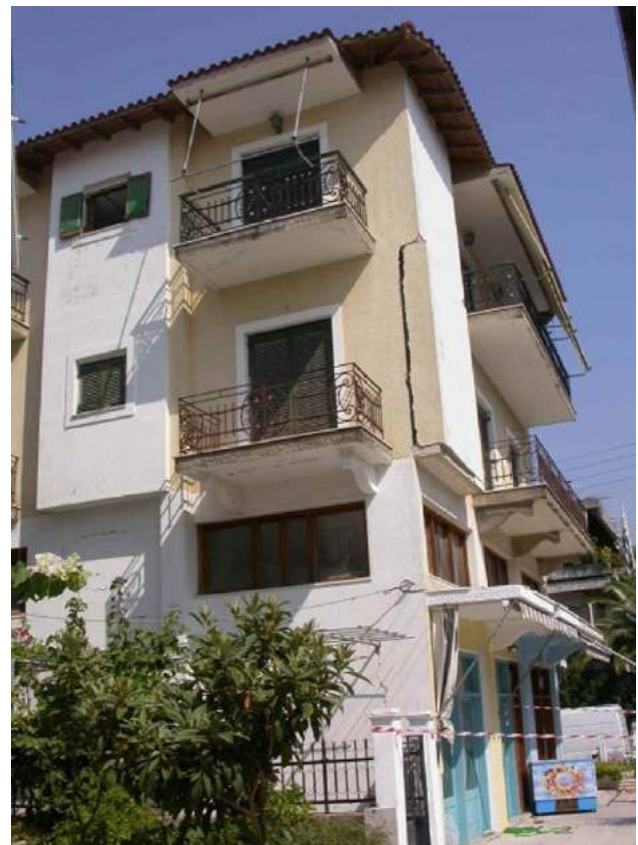
Fig. 13. Detachment of infill wall built out of the plane of the R/C structural frame. Architectural detail presenting a potential hazard in case of shaking.
