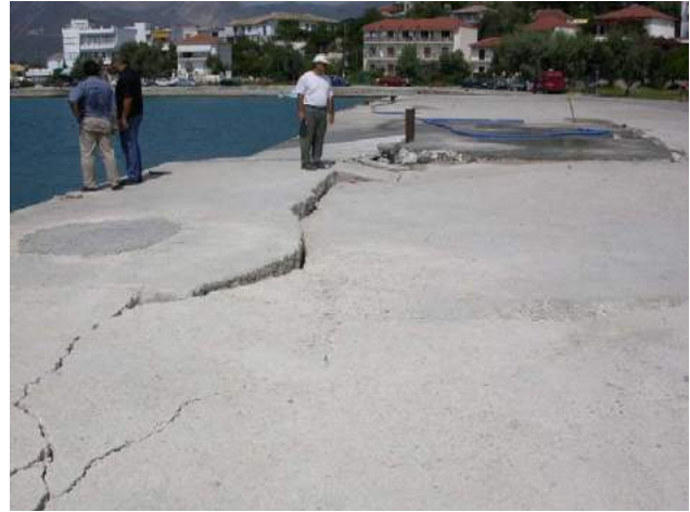
Fig. 3. Ground settlement and lateral spreading of poorly compacted fills behind the seawall in Vassiliki village caused cracking of concrete pavement.
