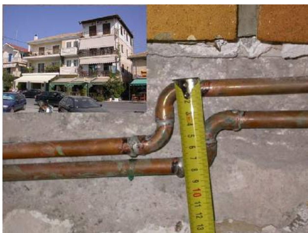
Fig. 5. Ground settlement resulted in 5 cm height difference between adjacent buildings in Lefkada waterfront, as witnessed by broken pipelines (photo taken after repair).
