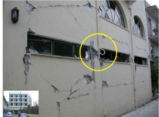
Fig. 12. Short column failure in R/C building (built in 1983).
