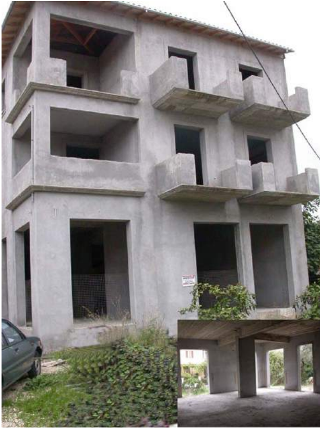
Fig. 17. A typical R/C building in the town of Lefkada that responded elastically during the mainshock. The inset photo shows the interior of the ground floor. Note the small spans of the beams and the extensive use of shear walls.
