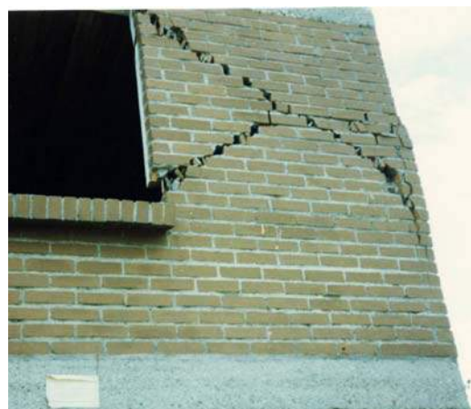
Figure 8. Shear failure due to wall stiffening.
