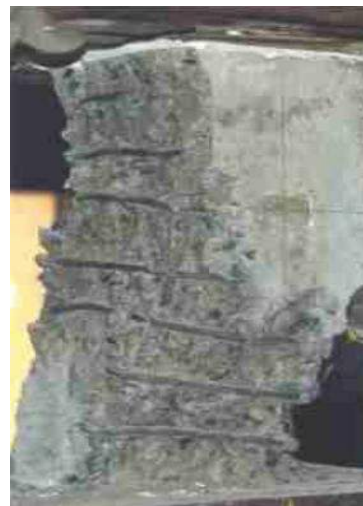
Figure 15. Concrete cover spalling and undamaged concrete core.
