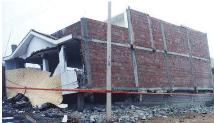
Figure 3. Collapsed house in the Atico earthquake.
