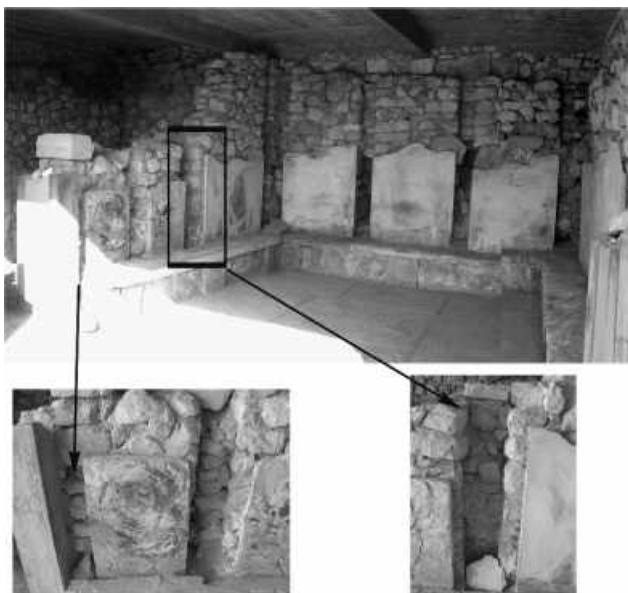
Figure 3. Villa in Ag. Triada, Room 4, northwest wing. Retaining wall with vertical timber reinforcement. The wall was covered with plaster elements. Timber elements were unplastered and, hence, protected from concentration of humidity (Tsakanika, 2006)
