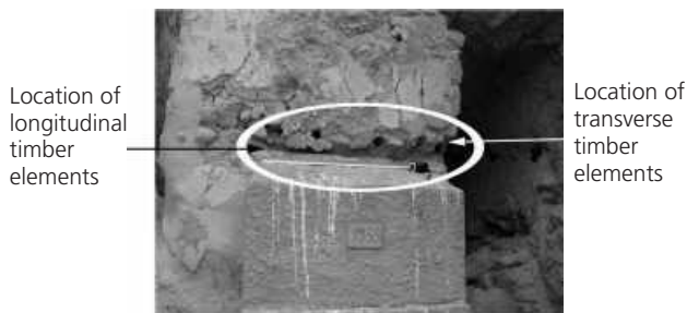
Figure 2. Old palace in Festos. Location of horizontal longitudinal and transverse timber elements in rubble stone masonry (Tsakanika, 2006)
