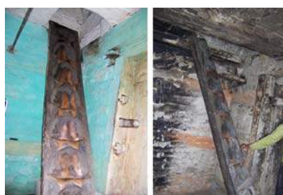
Figure 15. Ladders made of a single trunk used for access to upper floors.
