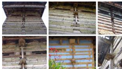
Vertical members ('shear keys') attached to the outer façade to prevent out-of-plane failure of the walls.
