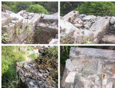
Figure 18. Detailing of the connection means at the wall corner. The horizontally placed wooden logs are connected by rectangular-shaped wooden pins. (Photographs show the rectangular holes foreseen at the log ends.)
