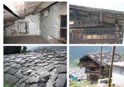
Figure 19. Detailing of the wooden roof construction and the roofing by large slate tiles.
