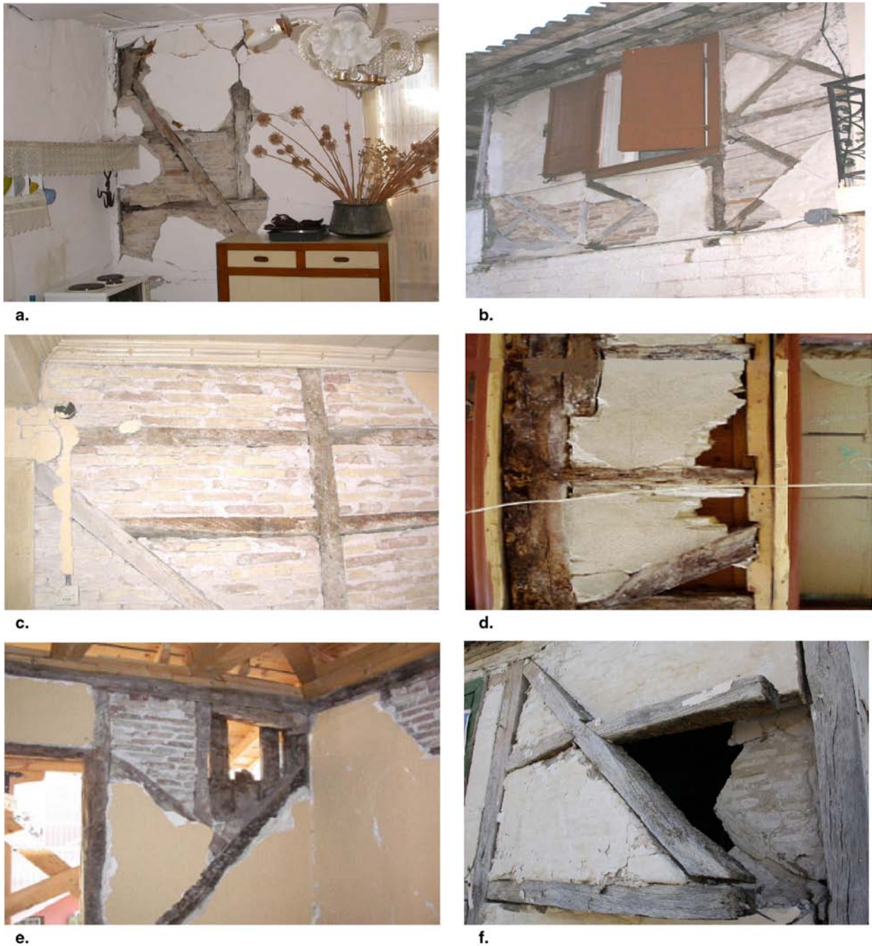
Fig. 8. a: Cracking of masonry walls at the ground floor. b: Failure of the plastered lime at the upper floor. c: Shear failure at the interface of wooden elements and masonry infill. d, f: Crushing of masonry infill at the corners of the wooden frame. e, f: Out-of-plane collapse of masonry infill.
