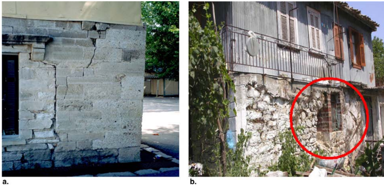
Fig. 7. a: Cracking of masonry walls at the ground floor. b: Local failure of masonry walls. Vertical loads from upper floor carried by the wooden frame on the ground floor.
