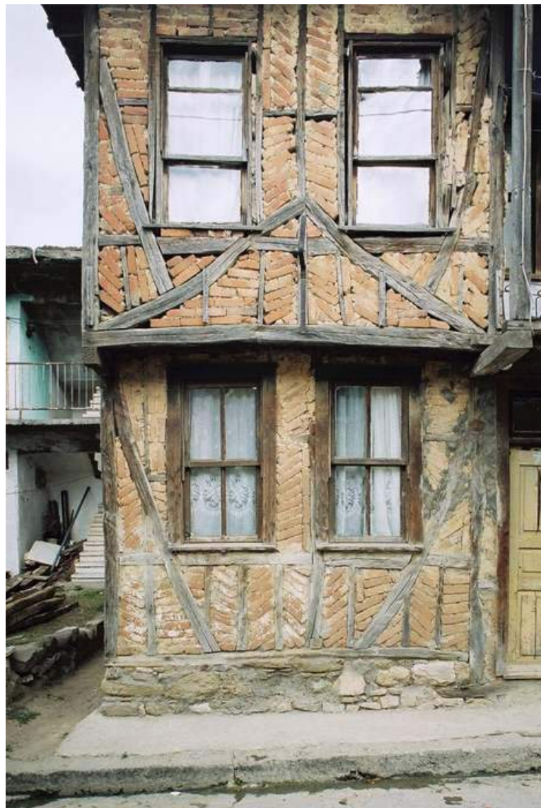
Figure 11: Himiş house in Gölcük after earthquake constructed in 1955. There was only slight damage to the interior of this house.
