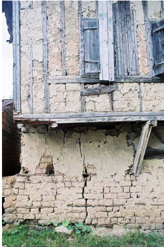
Figure 4: View of Infill-frame construction in the historic Ottoman town of Safranbolu, Turkey
