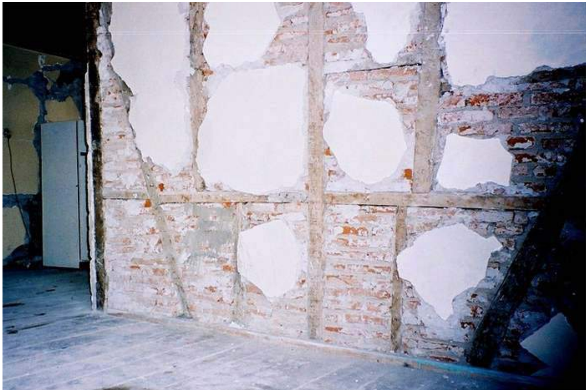
Figure 12: Hımsı interior wall in Düzce after earthquake.
