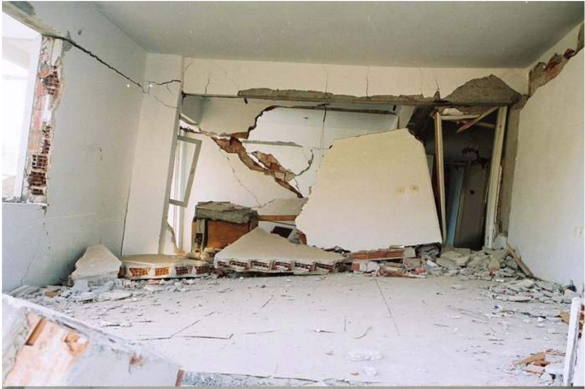
Figure 14: Collapsed interior infill wall in reinforced concrete building in Gölçük
