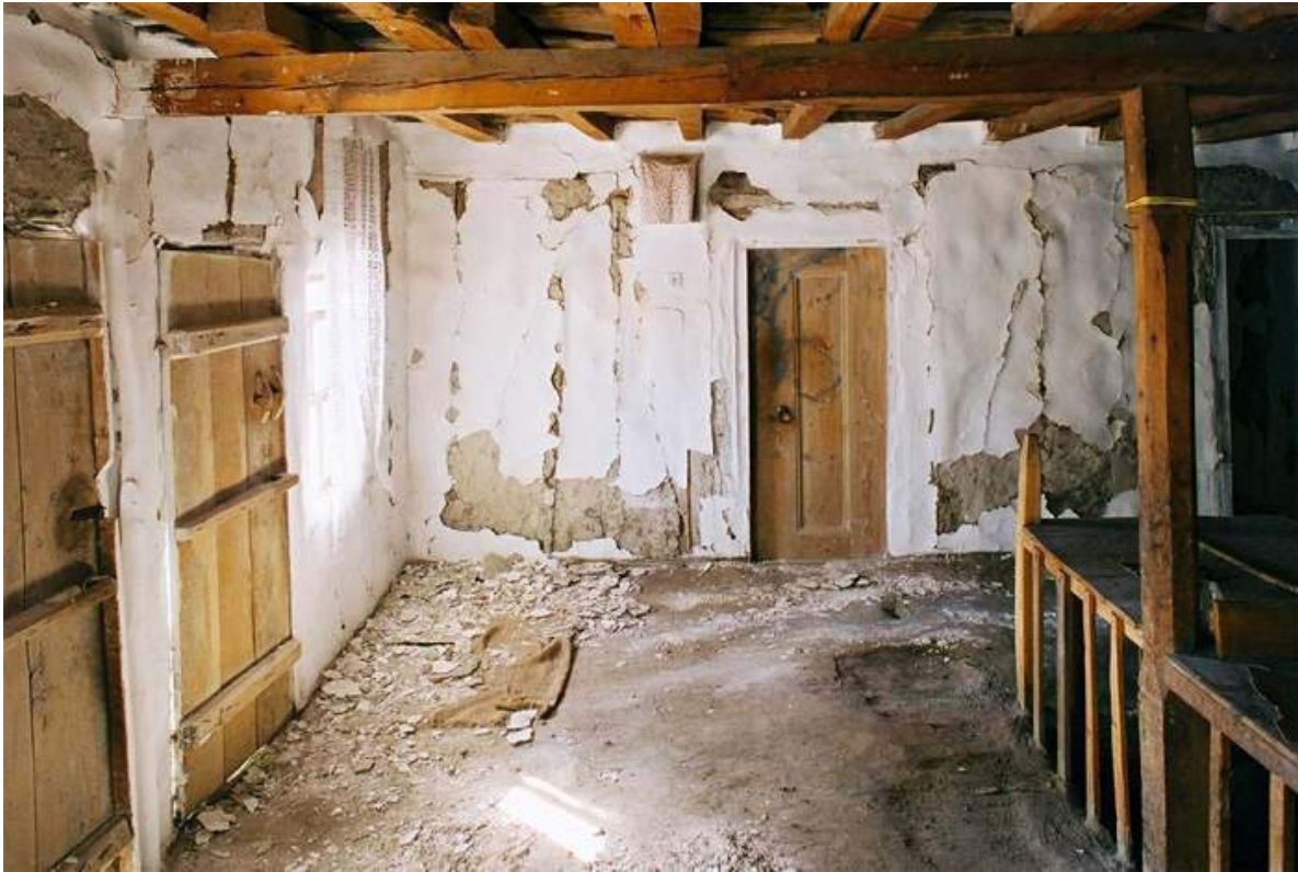
Figure 13: Interior of himiş house in Orta after earthquake showing damage to mud and lime plaster over infill walls.
