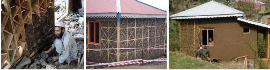
Fig. 2 Dhajji construction type in northern parts of Pakistan. From left to right construction of Dhajji wall, completed structure walls and completed Dhajji housing unit
