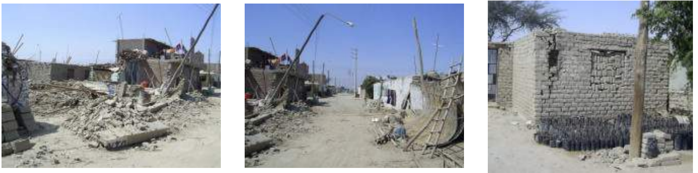
Figure 11. Traditional adobe houses with damage in Pachacutec
