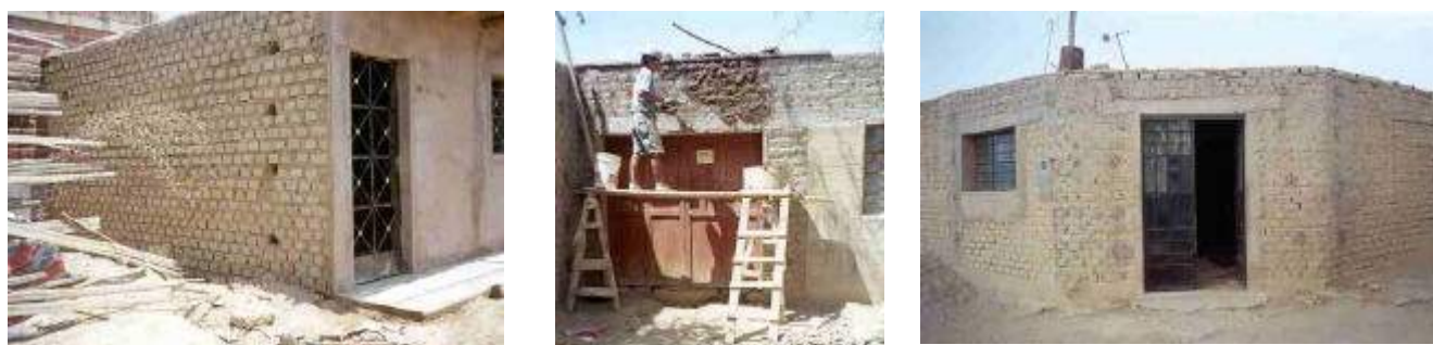
Figure 6. Demonstration adobe houses in (left to right) Ica Central, Parcona and La Tinguña, during reinforcement in 1998.
