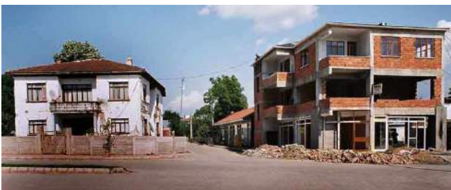
Figure 17: Three story RC building next to a 2½ story himiş house near Düzce showing the repair of severe damage to the RC building (notice the size of the ground floor columns). The himiş structure has lost only stucco on the side. Almost all of the hollow clay block on the RC building has been reconstructed after the earthquake. This shows that even low rise RC buildings sometimes suffered more damage than nearby traditional buildings.
