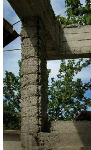
Figure 18: LEFT: House being reconstructed to replace one destroyed in Afyon earthquake. Concrete is being mixed on ground with garden hose and without slump test or measurements.
