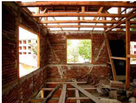
Figure 25 & 26: After witnessing the destruction of RC buildings around him in Duzce and seeing that his father's hımiş house survived undamaged, this resident of Düzce decided to stop building a new RC house and build a house for himself and his family with hımiş construction.
