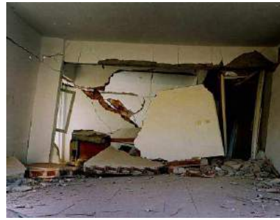
Figure 20: Hımış interior wall in house in Düzce earthquake damage district showing “working” of wall that caused loss of plaster.
