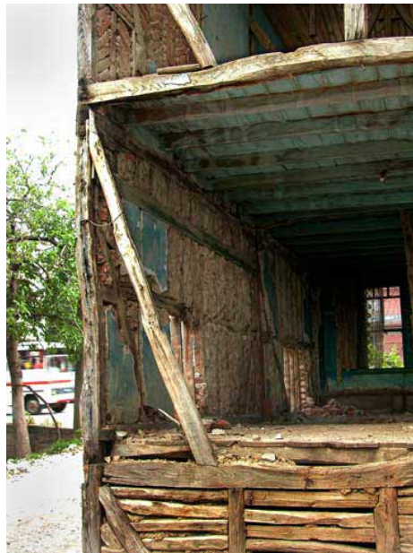
Figure 11 & 12: Partially demolished house in Golcuk showing the single brick wythe thickness of typical himış wall. On the LEFT is the exterior and on the RIGHT is the interior face of the same wall.
