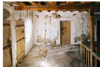
Figure 22: LEFT: House in Orta, Turkey one day after the 2000 Orta earthquake – showing plaster cracking that reveals the timber frame.
