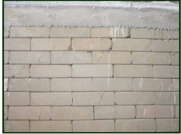
Figure 9: Wall 2, Typical block crack pattern
